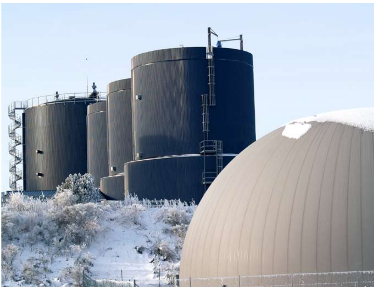
Large Danish Biogas plant (photo Biogassekretariatet)
